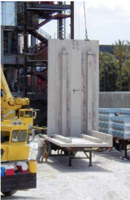
The 6-in.-thick x 22-ft-tall panels were reinforced with ribs spaced 6 ft apart.
