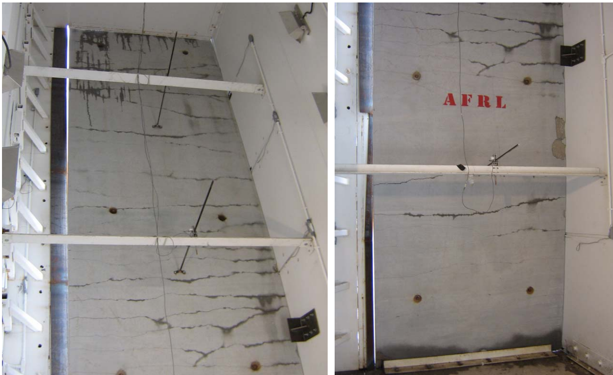
Figure 25: Internal View of Control Panel after Experiment 5
