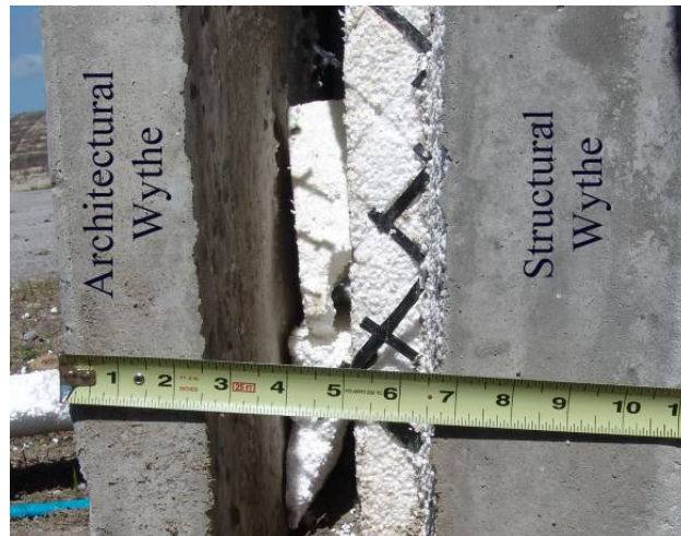
Figure 3: C-grid® wythe connection after testing (note section is damaged in photo due to loading)
