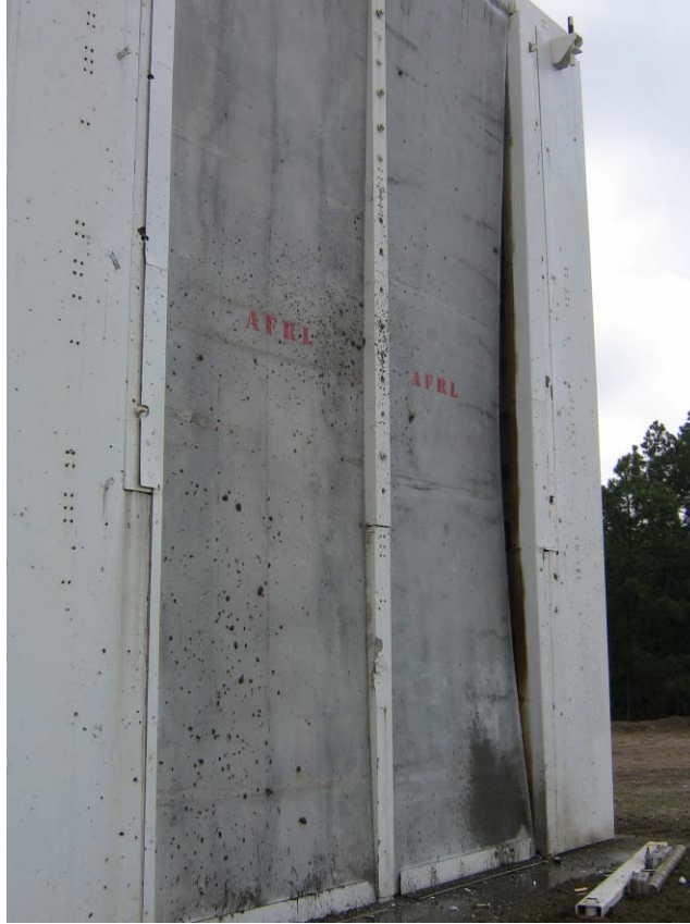
Figure 24: External View of Panels after Experiment 5
