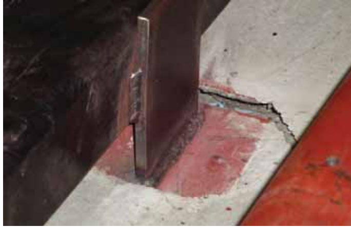
Figure 166. PCSD1-A Punching Failure of Connection
