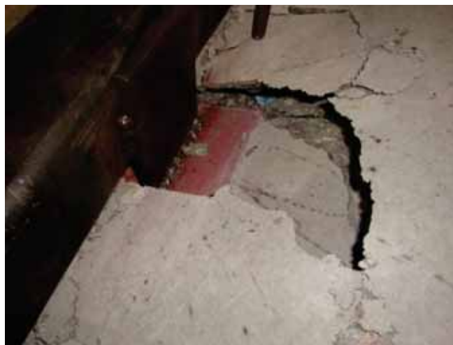
Figure 170. PCD1-C Punching Failure of Connection
