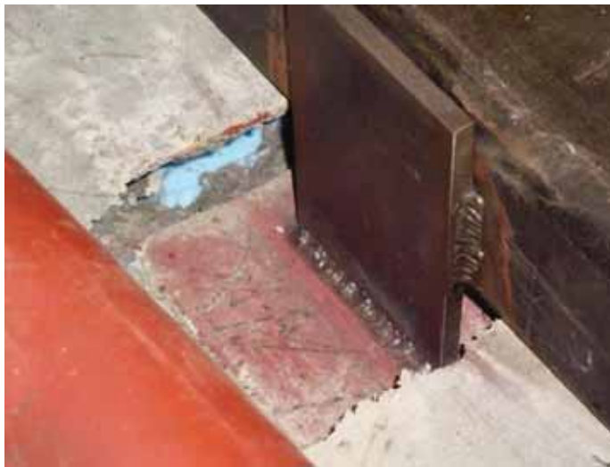
Figure 168. PCD1-B Punching Failure of Connection
